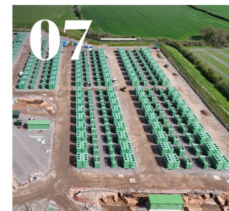
BW ESS: Scaling up the UK battery market
